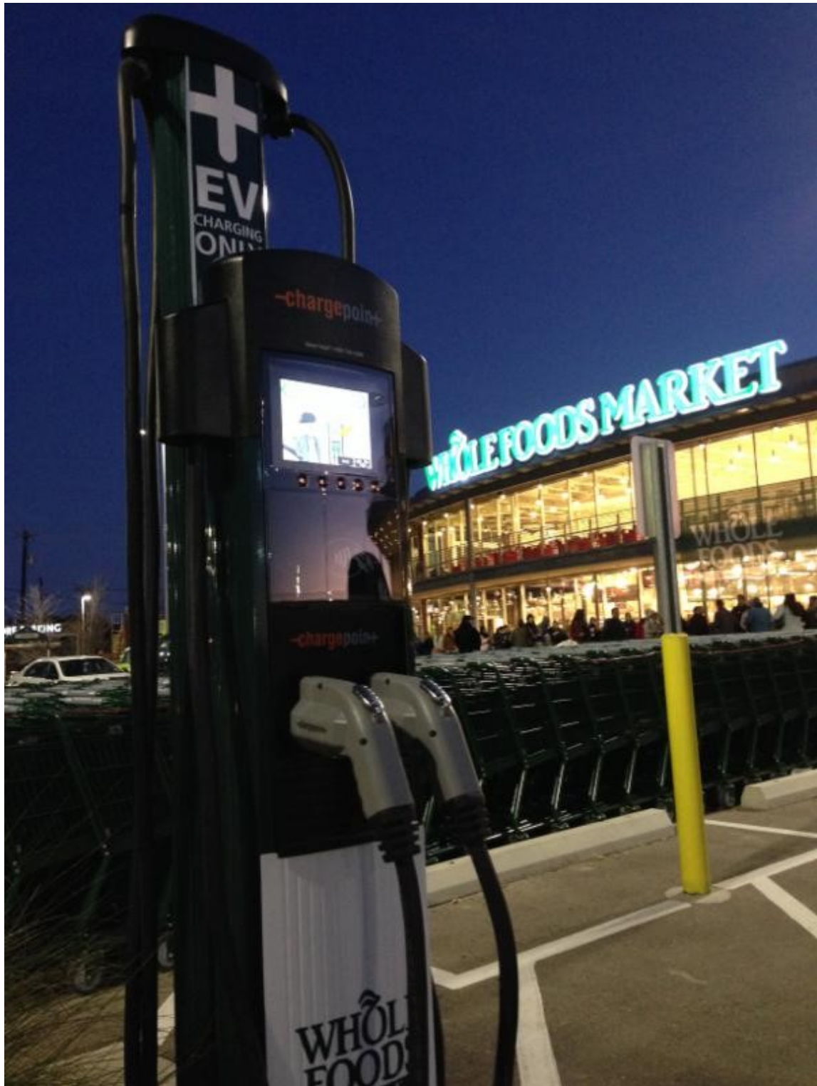
2015 - Level 2 EV Chargers at WFM
