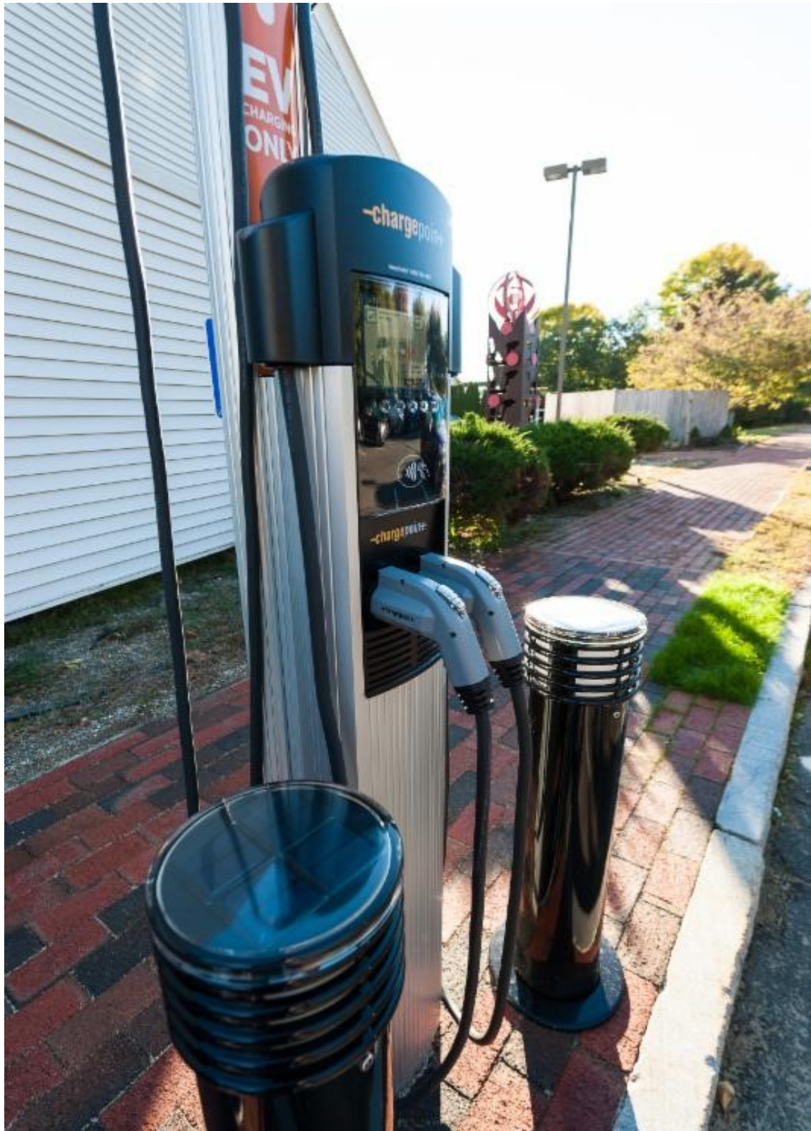
2015 - Level 2 EV Charger Madison CT
