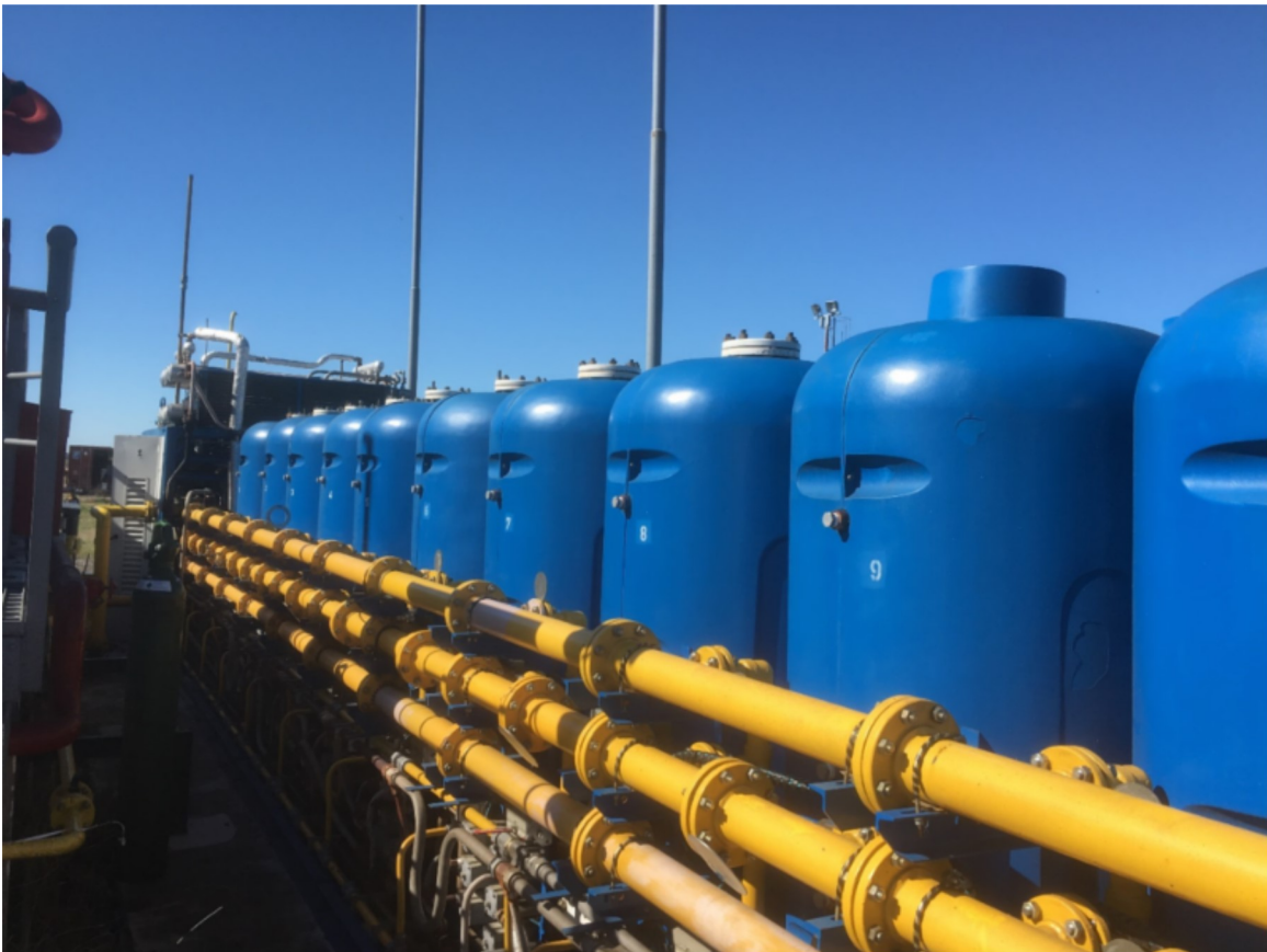
ZTPS-Biogas Treatment Plant
